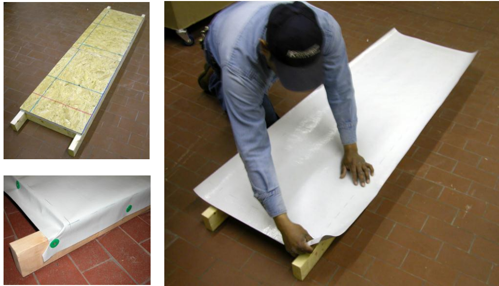
Figure 34. Photos of a technician wrapping a dehydrator ceiling panel with PolyMax fabric prior to installation.
