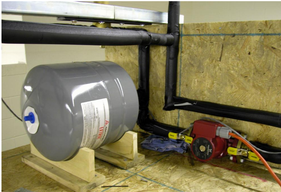
Figure 39. Continuous hot-water recirculation pump; also shows expansion tank.
