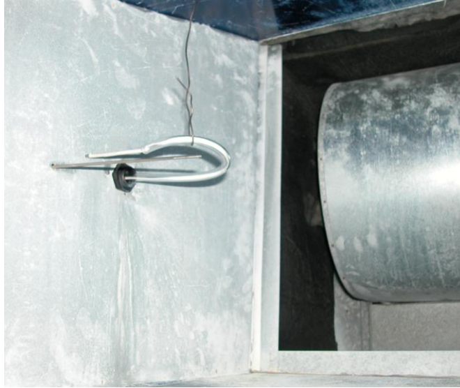
Figure 52. Dry (foreground), and wet bulb thermocouples, and water wick viewed inside the air ductwork. The fan shroud for the hydronic heater is visible in the background.
