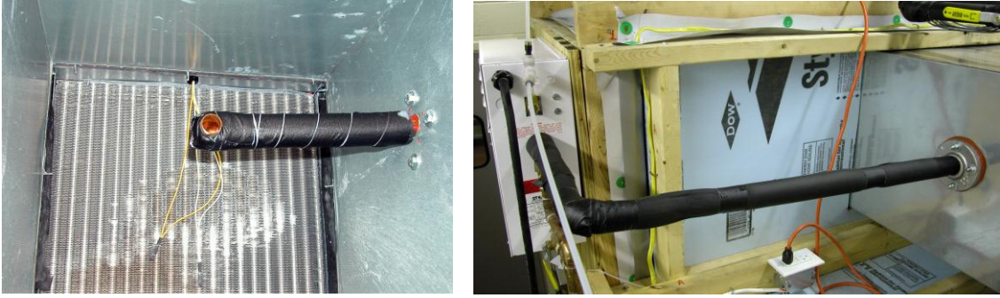
Figure 48. Steamist steam generator discharge piping. Left photo shows pipe discharge inside of duct, right photo shows piping from generator to duct
