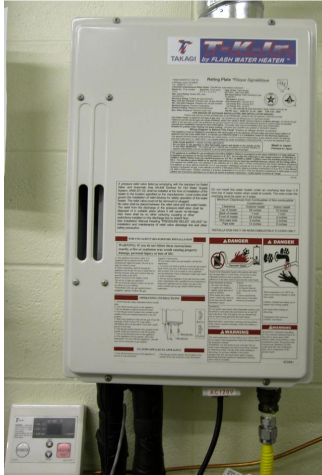
Figure 29. Continuous hot water heater and temperature controller mounted on wall adjacent to dehydrator.
