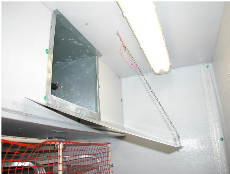
Figure 44. Air deflection baffle mounted parallel to and adjacent to the bottom side of the heated air discharge duct. The angle shown is 15 degrees below horizontal. The baffle serves to direct the heated air to the low pressure side of the LSHV fan.
