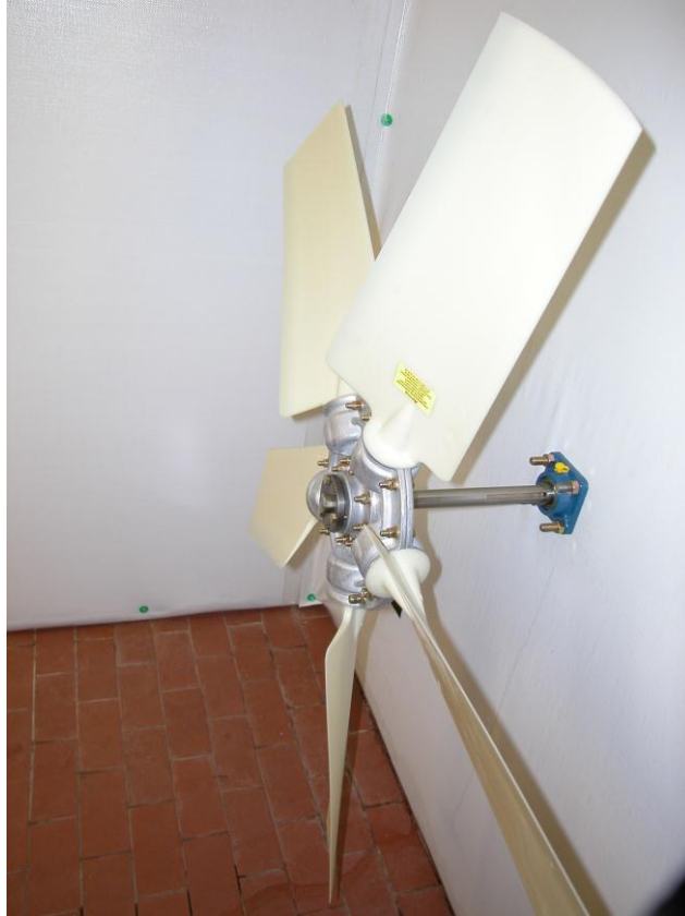
Figure 42. Low-speed, high volume fan installed to mix air within the dehydrator.
