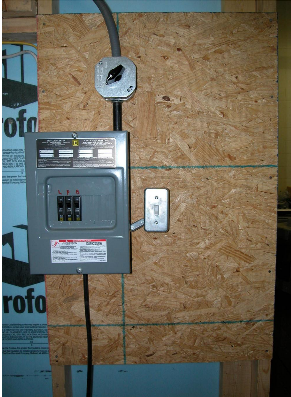
Figure 37. Electrical enclosure mounted on the left-hand side of the dehydrator
